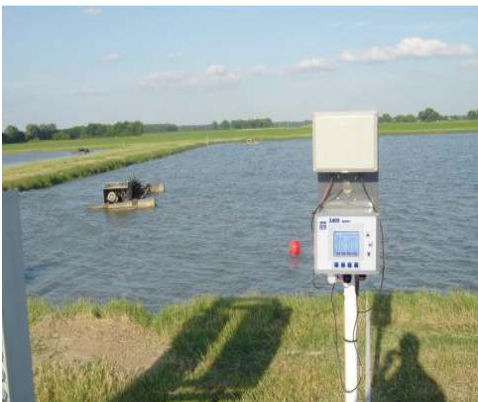
A 5400 deployed pond-side to control paddle wheels
